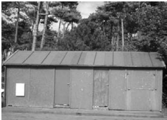
The clubhouse in its original state of disrepair
